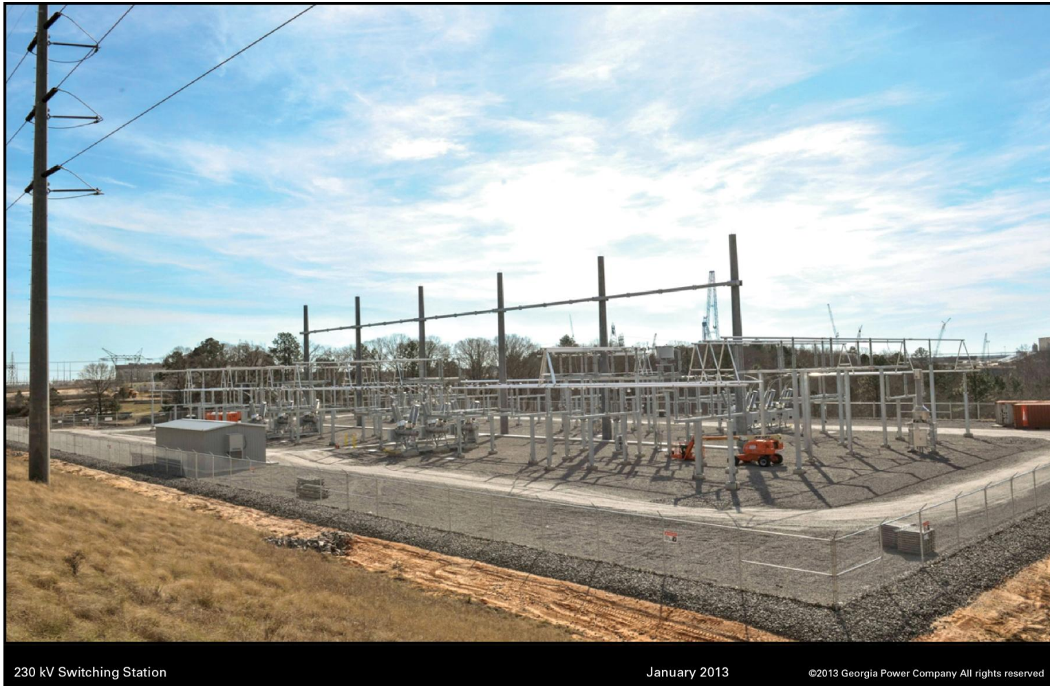
Photo 8 – Vogtle Unit 3 and 4 Switching Station
